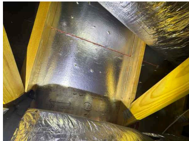
Attic Ventilation: Static Exhaust Port, Slope Vent
