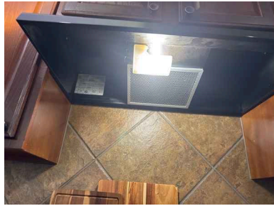
Range Exhaust: Vents to Exterior
