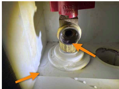
Washing machine connection
