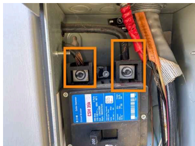
Main electrical panel
