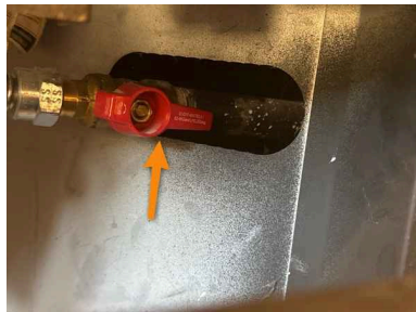
Gas valve turned on
