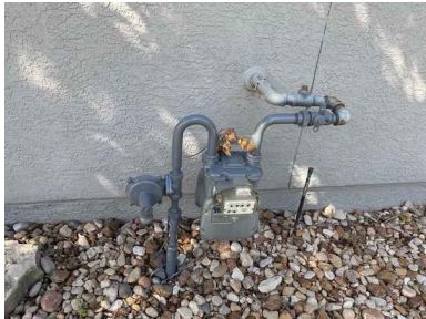
Gas Meter Bonded at Meter: Yes
